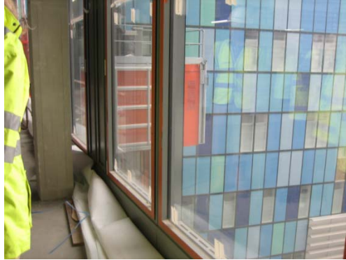
15/5/2009 Outside lift IMG_3951.jpg
