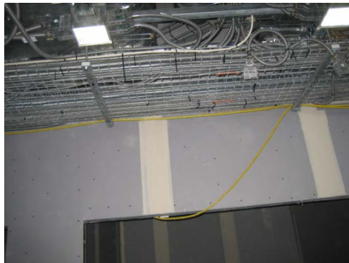
15/5/2009 Further down: wires for IT IMG_3956.jpg
